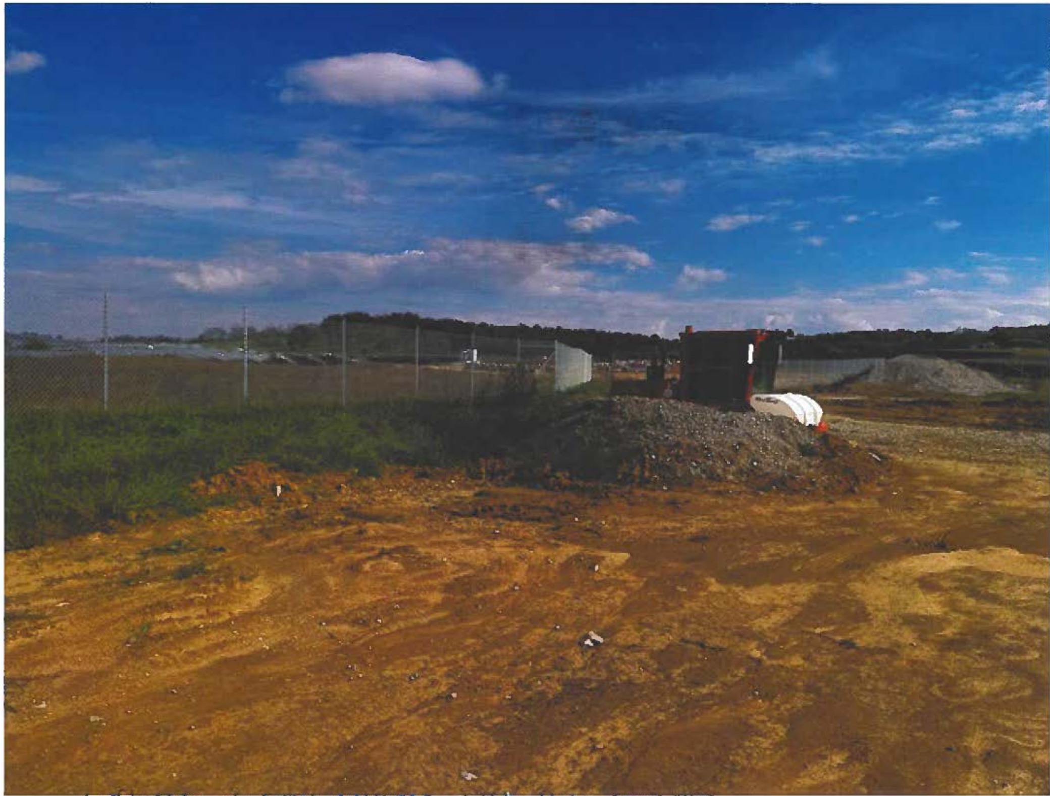
Left side of front entrance. Dirt, Ruts. Gravel Pile
