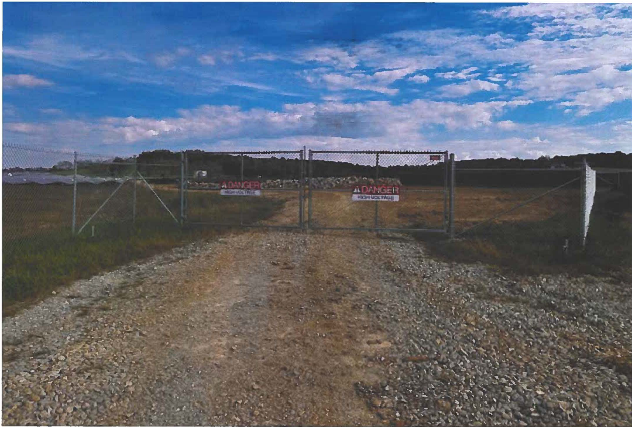
The entrance. Ruts. Mud. Dirt. Insufficient Gravel.
